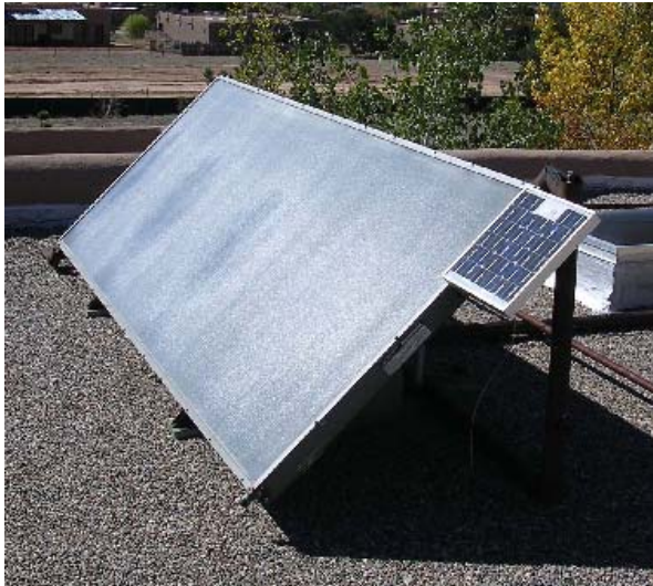
Domestic Solar Hot Water
