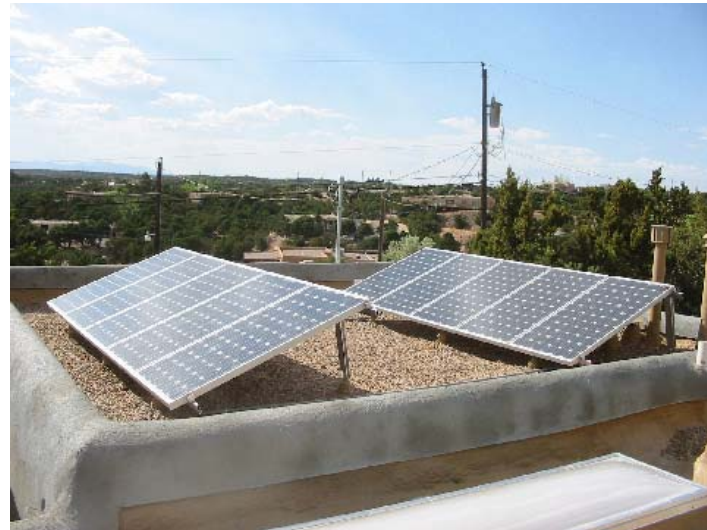
Grid-tied Solar Electricity (PV)
